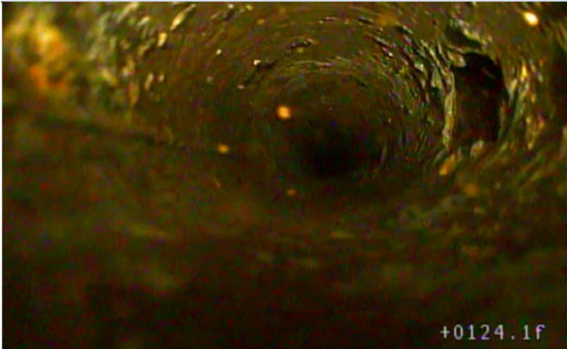
Figure 2: Riverbank Well No. 10 Transducer Pipe Corrosion Hole (Source: BEEST, Inc. Video Camera Survey Report, March 24, 2022)
