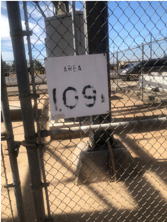
Transformer West of Building 13 – View toward West 17 SEPTEMBER 2025
