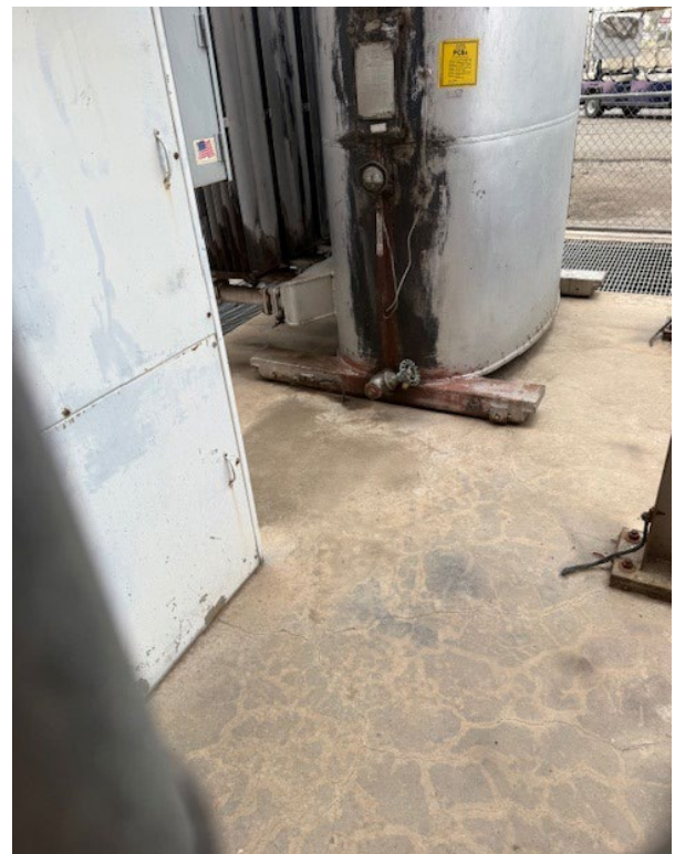
Substation 18 – View toward Southeast 18 SEPTEMBER 2025
