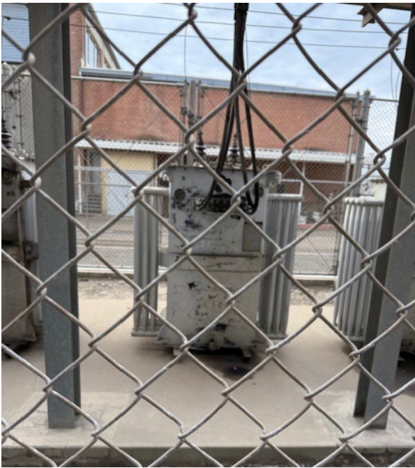
Substation 14 (center transformer) – View toward South 18 SEPTEMBER 2025
