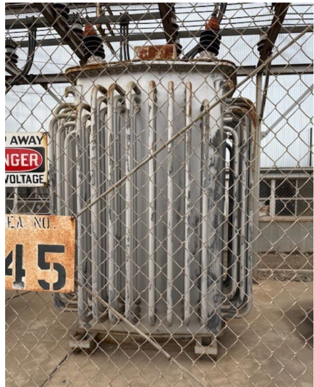
Substation 17 (center transformer) – View toward South 18 SEPTEMBER 2025
