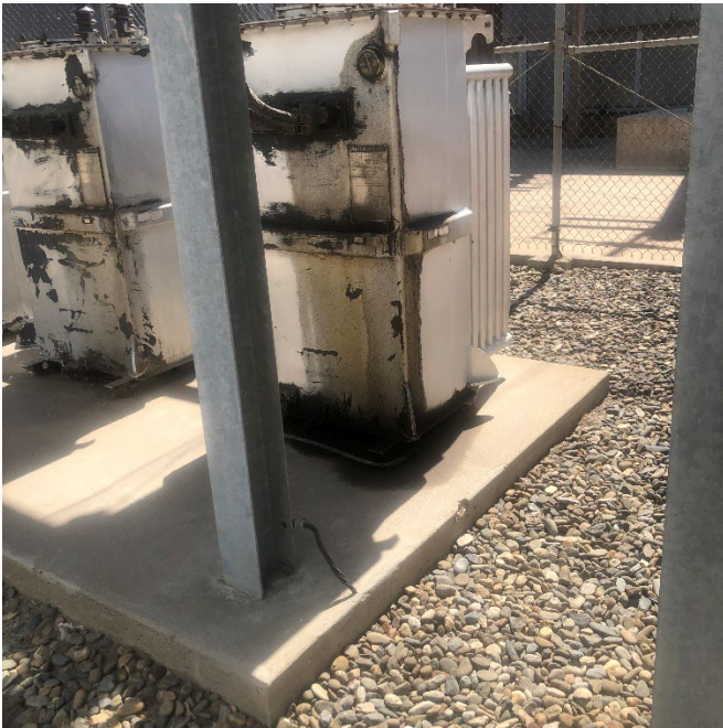
Substation 4 – View toward Southwest 17 SEPTEMBER 2025
