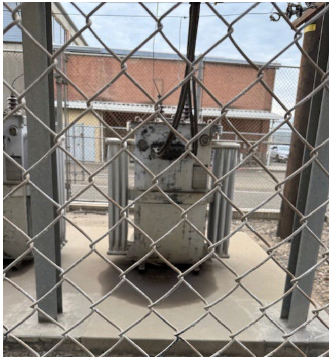
Substation 14 (west transformer) – View toward South 18 SEPTEMBER 2025
