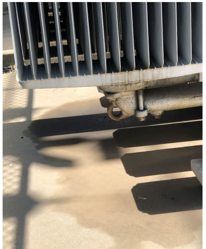
Substation 12 – View toward West 17 SEPTEMBER 2025
