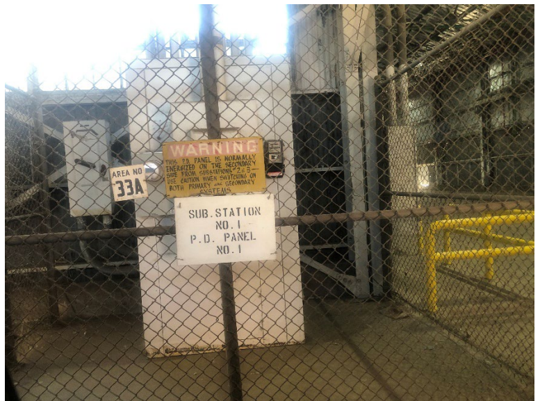
Substation 1 – View toward East 17 SEPTEMBER 2025
