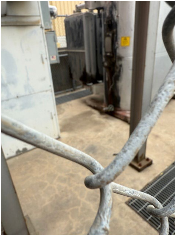
Substation 18 – View toward Southeast 18 SEPTEMBER 2025
