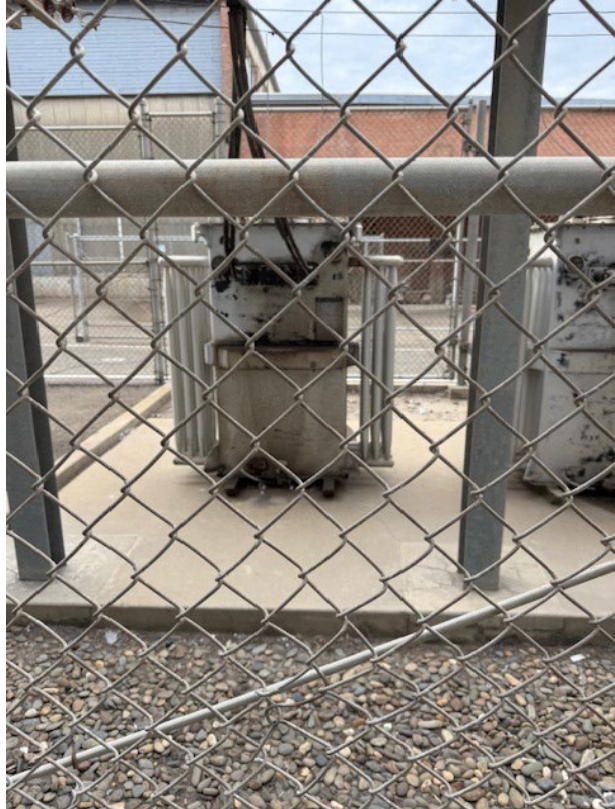
Substation 14 (east transformer) – View toward South 18 SEPTEMBER 2025
