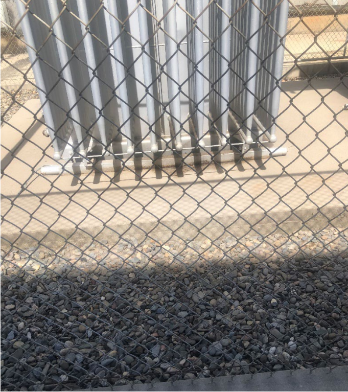
Substation 7 – View toward North 17 SEPTEMBER 2025
