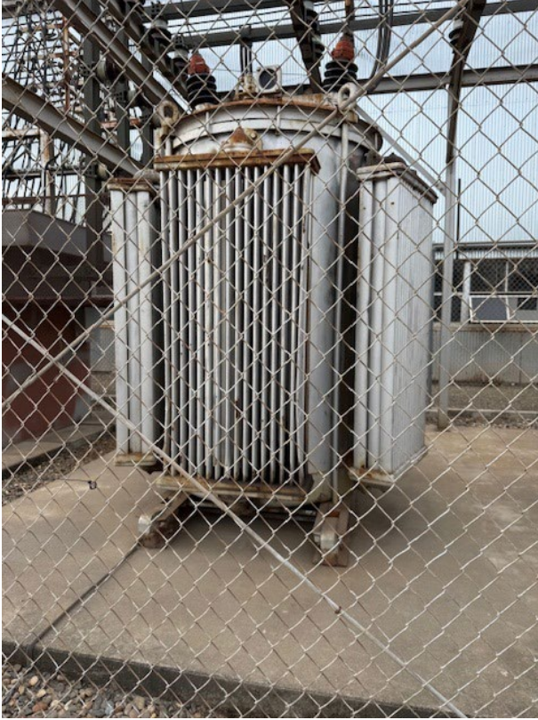
Substation 17 (east transformer) – View toward South 18 SEPTEMBER 2025
